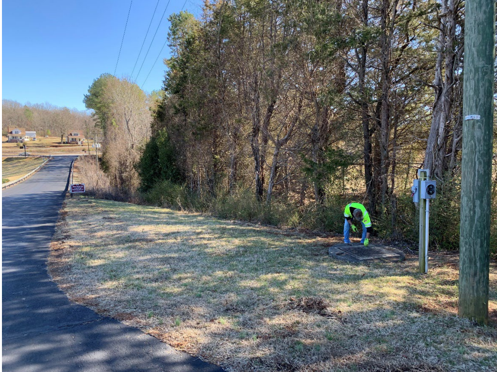
Existing Inactive Meter Vault (tie-in location)
