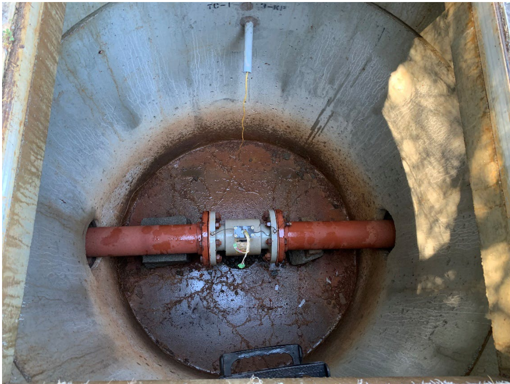
Existing Meter Vault on School Property
