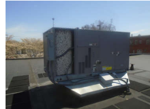
Existing AHU at the Martin Bldg. showing coil fins with extreme damage from hail.
