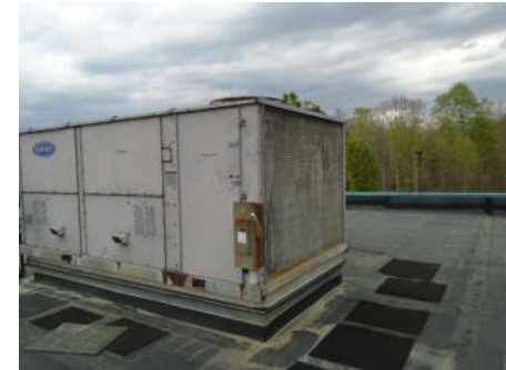
Existing AHU serving HSB. Units are over their useful life and are in need of replacement. Units shown to have similar hail damage at coil fins.
