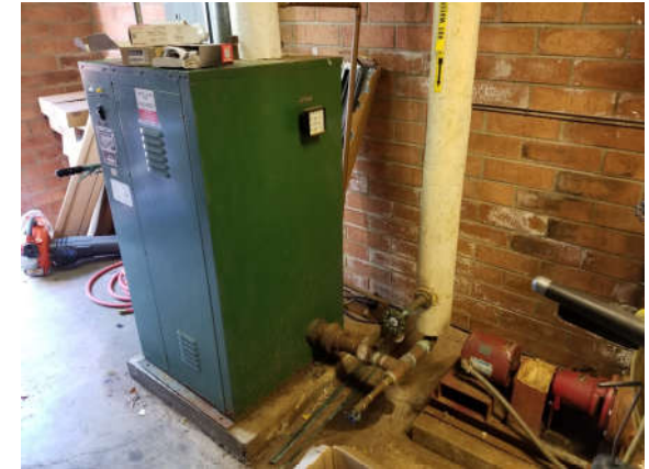
Existing electric boiler serving the Martin Administration bldg.
