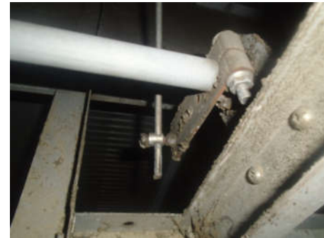
Existing actuator rod at IGV, currently broken.
