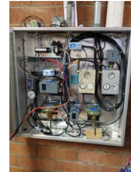
Pneumatic System at Martin Admin.
