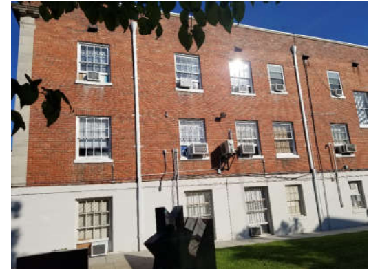
Back side of the Moses Bldg with existing single pane windows and AC units.
