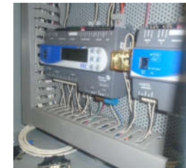
JCI Metasys Control System at the Courthouse.
