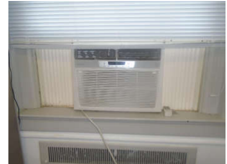
Example of existing Window AC units and Steam Radiators at Moses.
