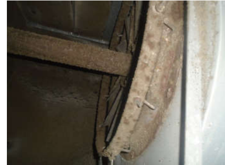
Existing inlet guide vane at AHU-2.
